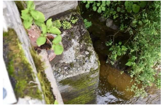
橋台天端の断面欠損
